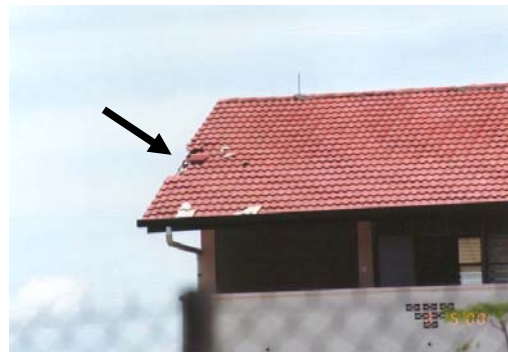
Figure 10: Photograph of a stricken point on the slanting edge of the gable roof. The air terminal conductor should also be installed on the edges of the gable roof.
