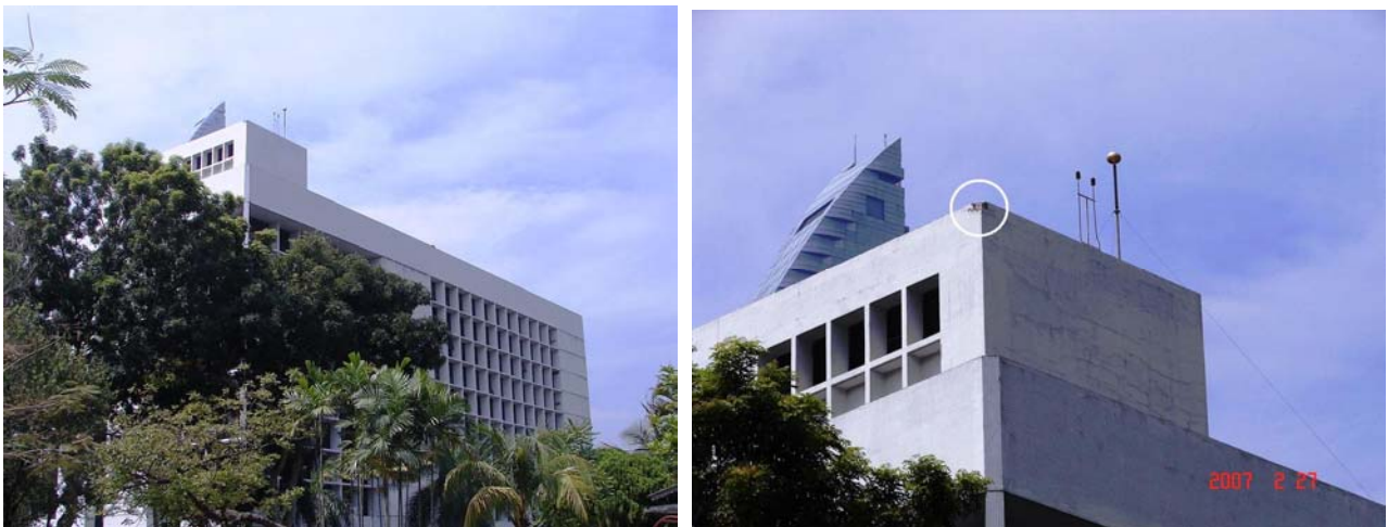
Fig. 2 – A bypass occurred close to a CVM air terminal that is positioned according to the proprietary collection volume method.
