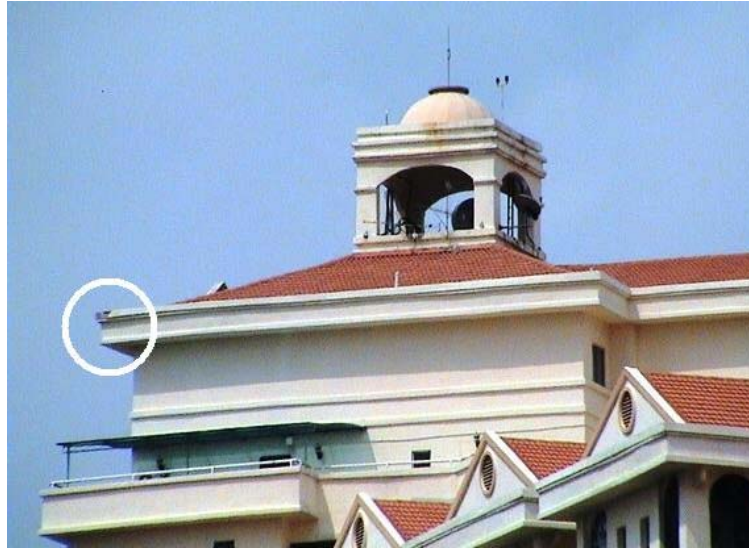
Fig. 5 – The bypass that occurred at the corner of the South-East tower block. This bypass is similar to that shown in Figs. 1 and 2.
