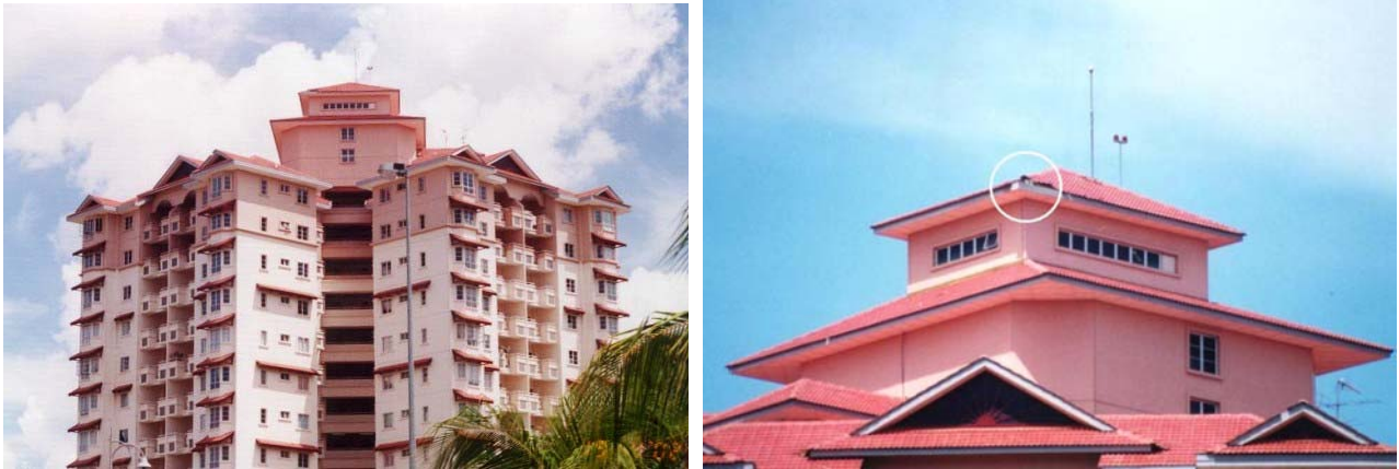
Fig. 1 – A bypass occurred close to an ESE air terminal that is manufactured and positioned according to the NFC 17-102 standard.
