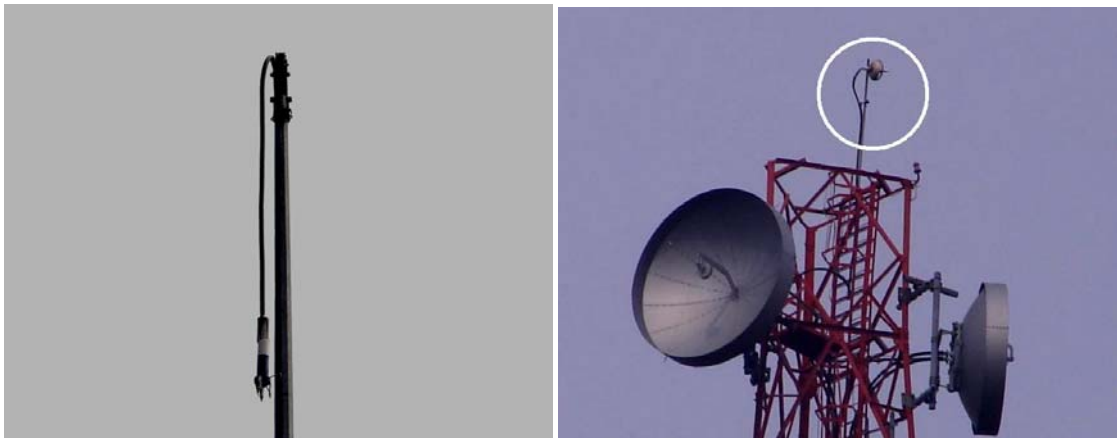
Fig. 13 – Photographs showing the ESE (left) and CVM (right) air terminals hanging by their down conductors as a result of damages to their non-metallic mounting poles.
